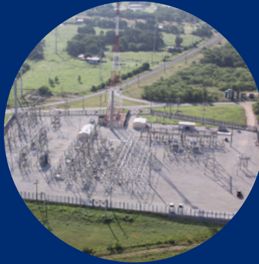
Access points outside substations
