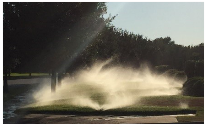
Figure 3. An example of sprinkler heads operating at high pressure, resulting in misting.
