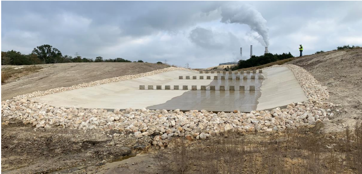
PHOTO 1 – View of new CBL Channel Discharge Structure at the CBL Pond (11-13-2020)
