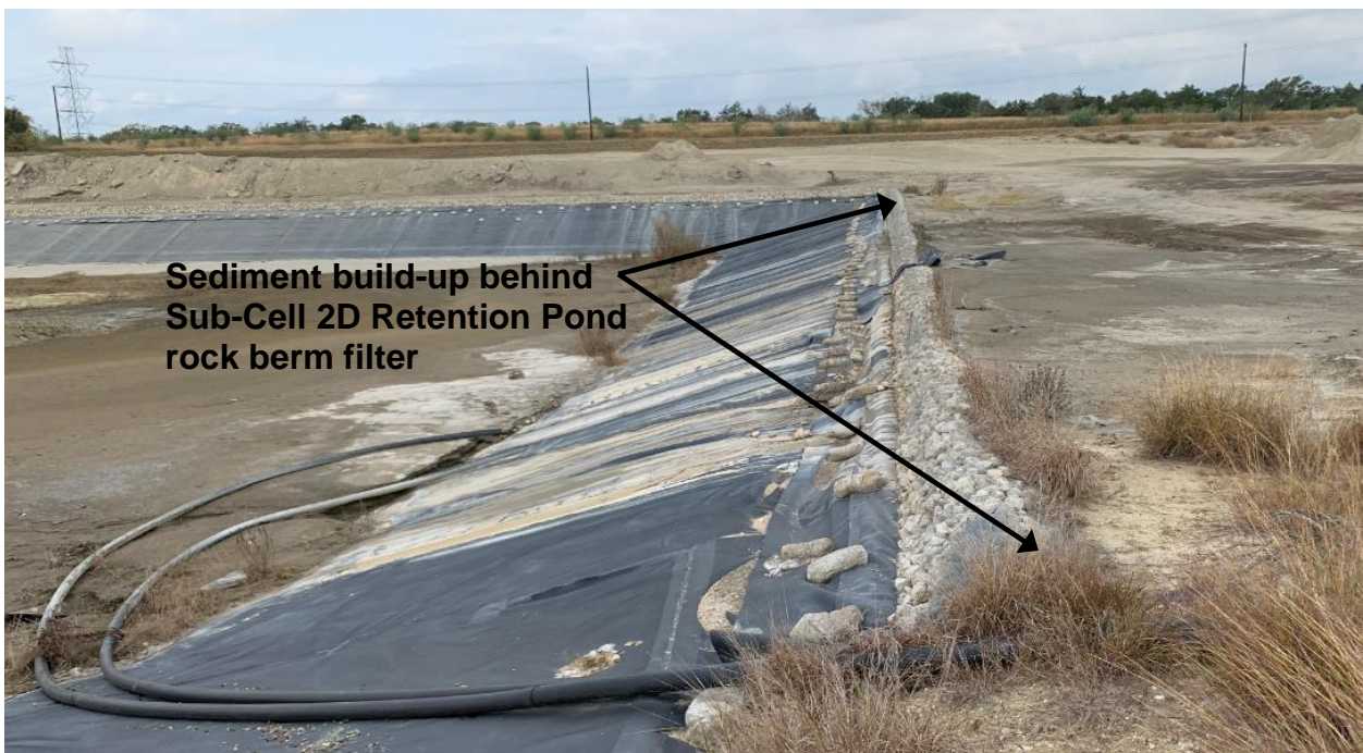
PHOTO 2 – View of excessive sediment build-up behind rock berm filter (11-13-2020)
