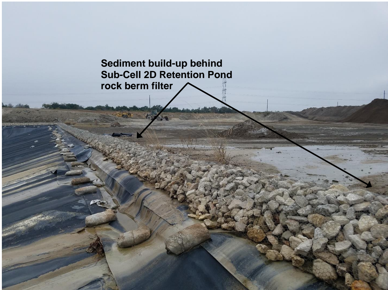
PHOTO 5 – View of excessive sediment build-up behind rock berm filter (11-07-2019)
