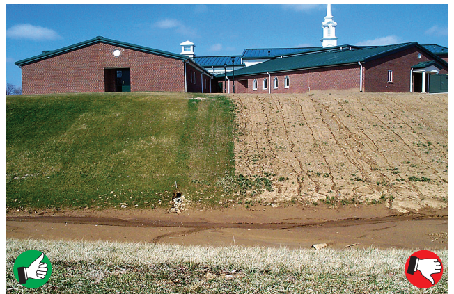
Erosion and sediment loss is virtually eliminated on seeded areas (left side). Rills and small gullies form quickly on unseeded slopes (right side).
