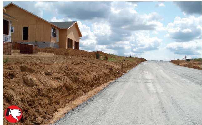
This residential management site shows poor management of bare soil areas. No erosion and sediment controls are present, and the grade on the existing slope is inadequate. Temporary or permanent seed, sod or mulch must be applied as soon as final grade is achieved. No slopes steeper than 3:1 are recommended.
