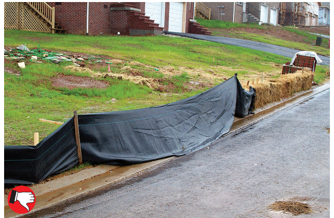
Poor installation of silt fencing, fair to good seeding. Silt fence must be trenched in along bottom and include wire backing. Straw bales are not approved as sediment barriers.
