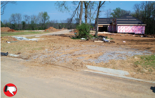
Poor construction entrance. Rock pad is poorly constructed; rock is too small. Use filter fabric under rock and larger sized rock, such as 3-5 inches. No mud should be tracked onto paved roads open for traffic.
