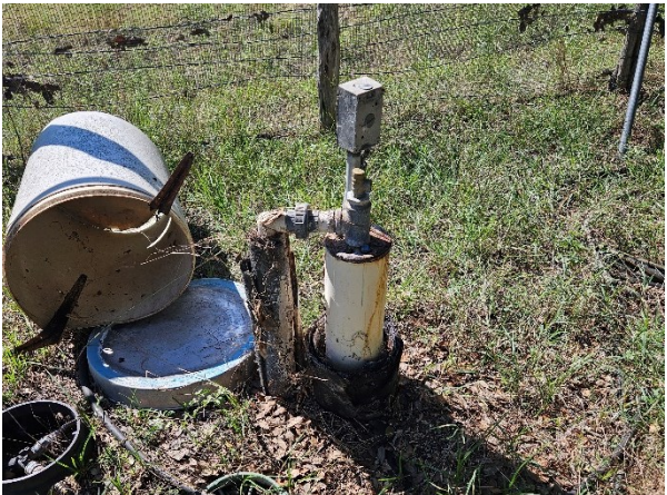
S-3: Water Well
