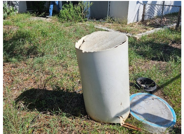
S-3: Water Well with Cover
