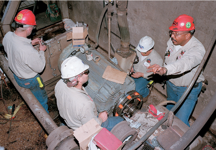
Employees at the Fayette Power Project and other LCRA power plants work 24 hours a day, 365 days a year to generate electricity for more than 1 million people in Central Texas.
