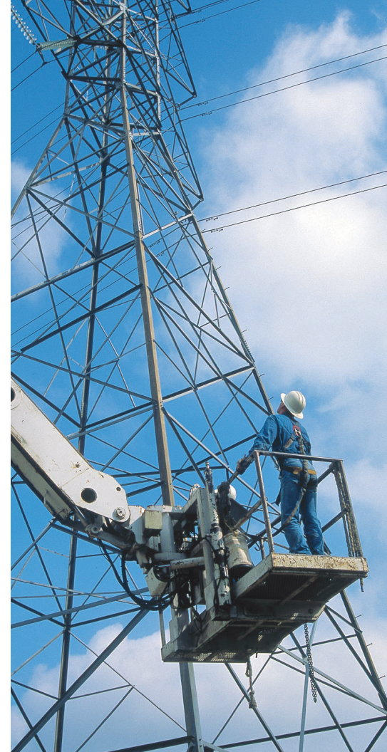
LCRA employees regularly inspect and maintain more than 3,300 miles of transmission lines and equipment in 53 counties across Central Texas.
