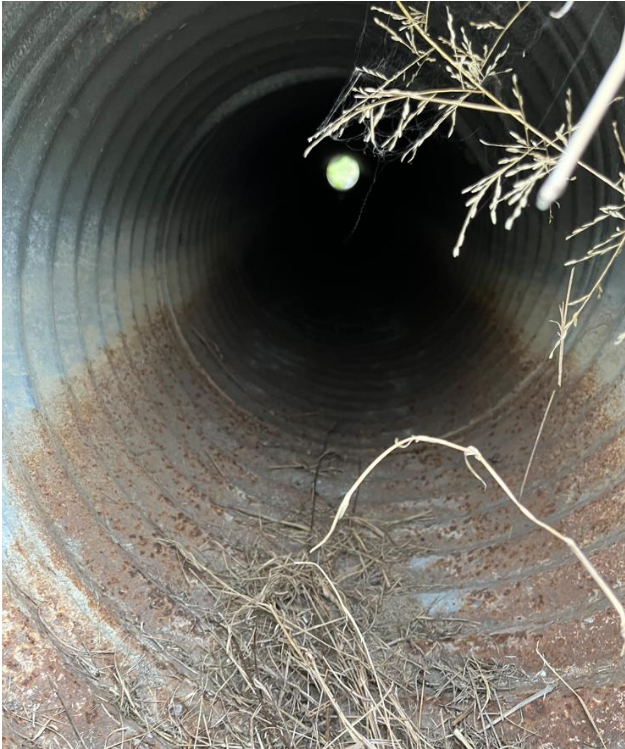
PHOTO 3 – View of Properly Functioning Non-Contact Water Drainage Culvert Pipe at Northeast Corner of Cell 1 (12-01-2022)
