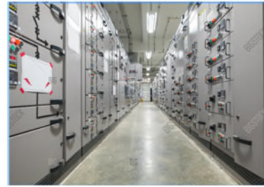
Figure 3 Switchgear Room 1 Lot can cost $153,000
