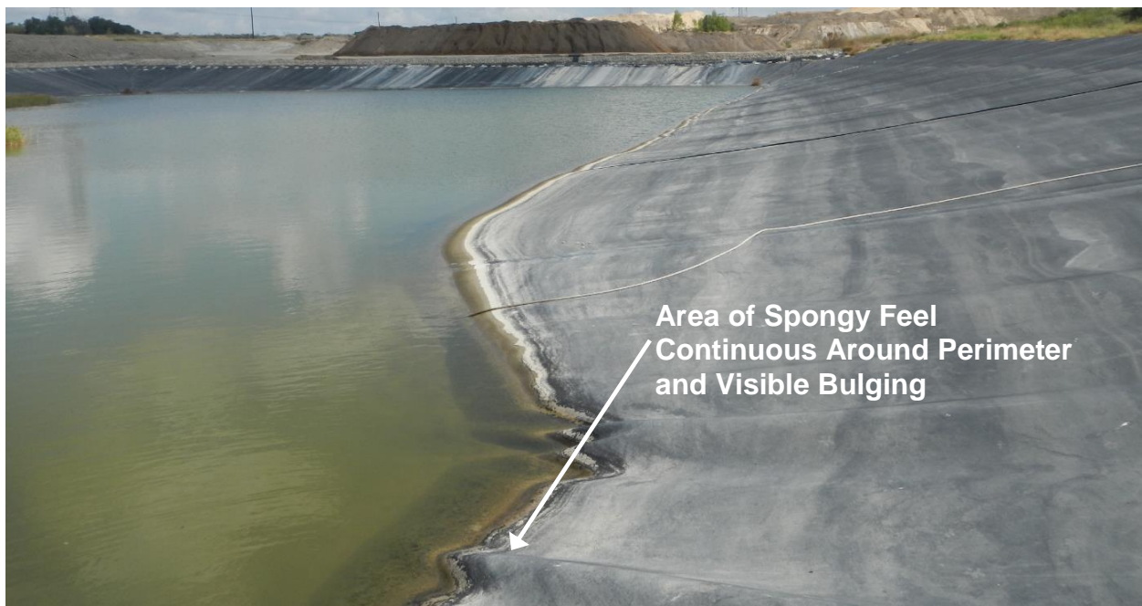
PHOTO 2 – View of Cell 2D Pond HDPE liner looking west at the Northeast corner (8-16-2018)
