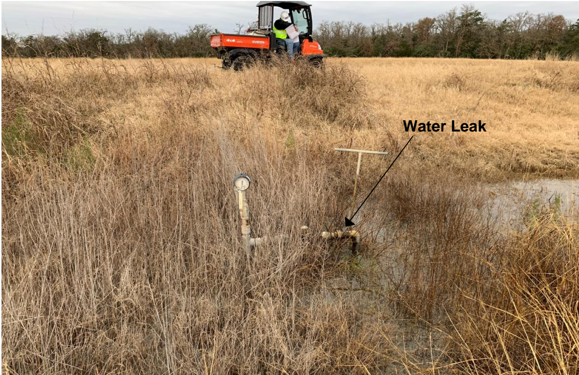
PHOTO 1 – View of leaking water meter upstream side of the West Embankment (12-12-2018)
