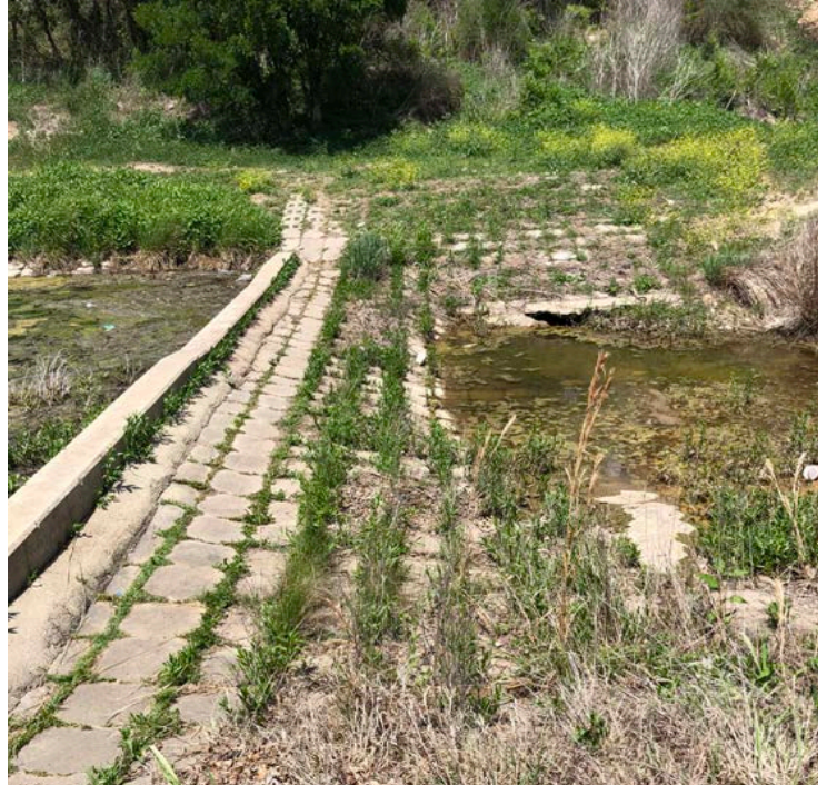
Small channel dam installed in Brady Creek to increase dissolved oxygen. There are multiple perforations on the downstream slope of the dam that help to aerate the water during base flow conditions.
