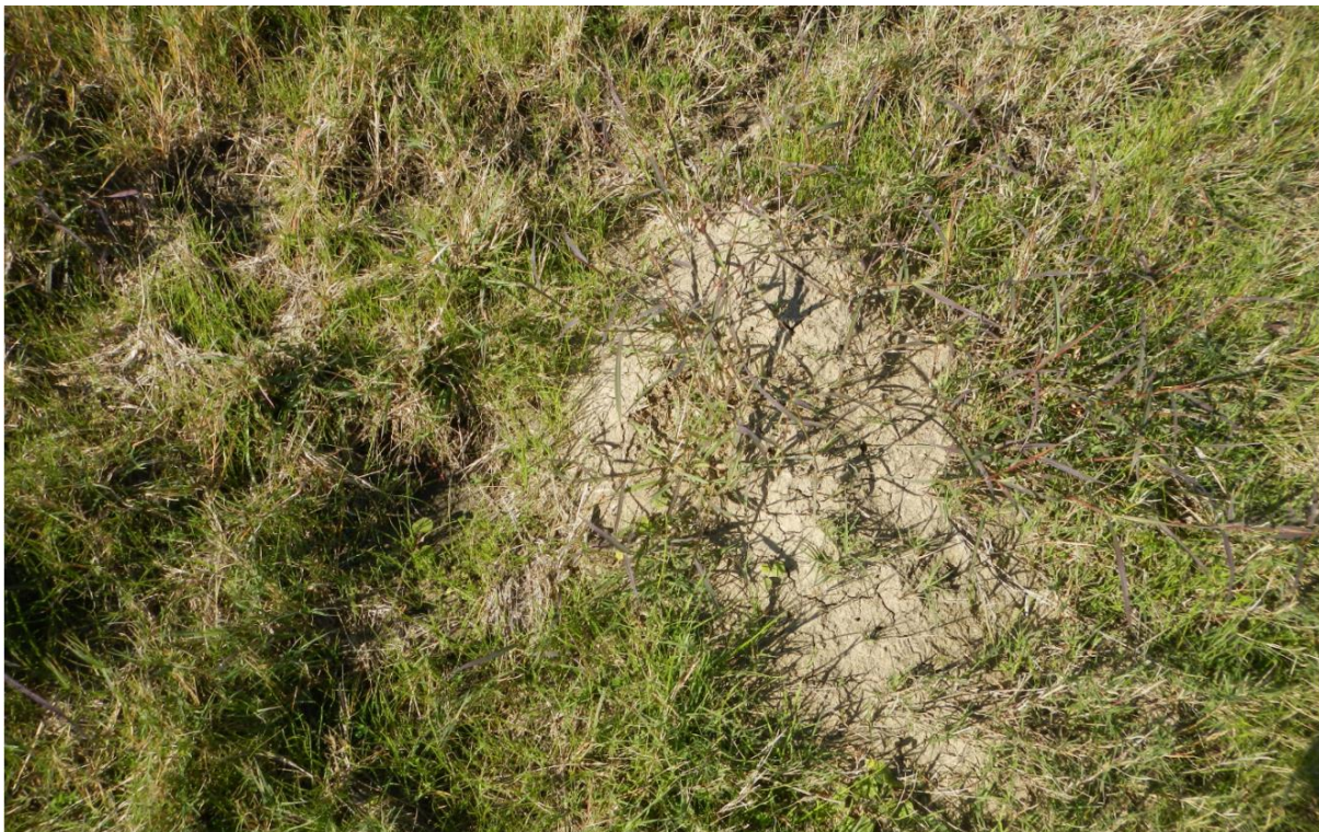
PHOTO 6 – View of Ant Mound and Evidence of Surface Drainage on the North End of East Embankment Slope Near the Crest (12-09-2015)
